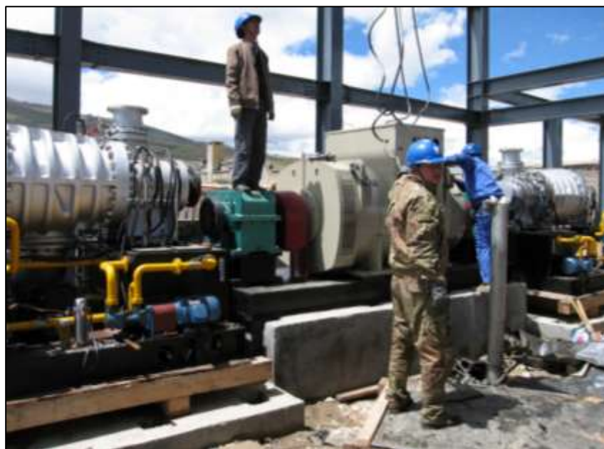
Figure 1 - 1,000 kWe screw-expansion engine installed in Yangbajain geothermal power station in Sep. 2008
