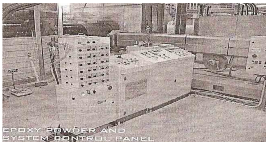
Figure 3 – View of epoxy controller
