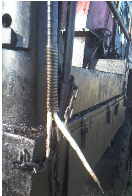
Figure 5. Cable break at a well
