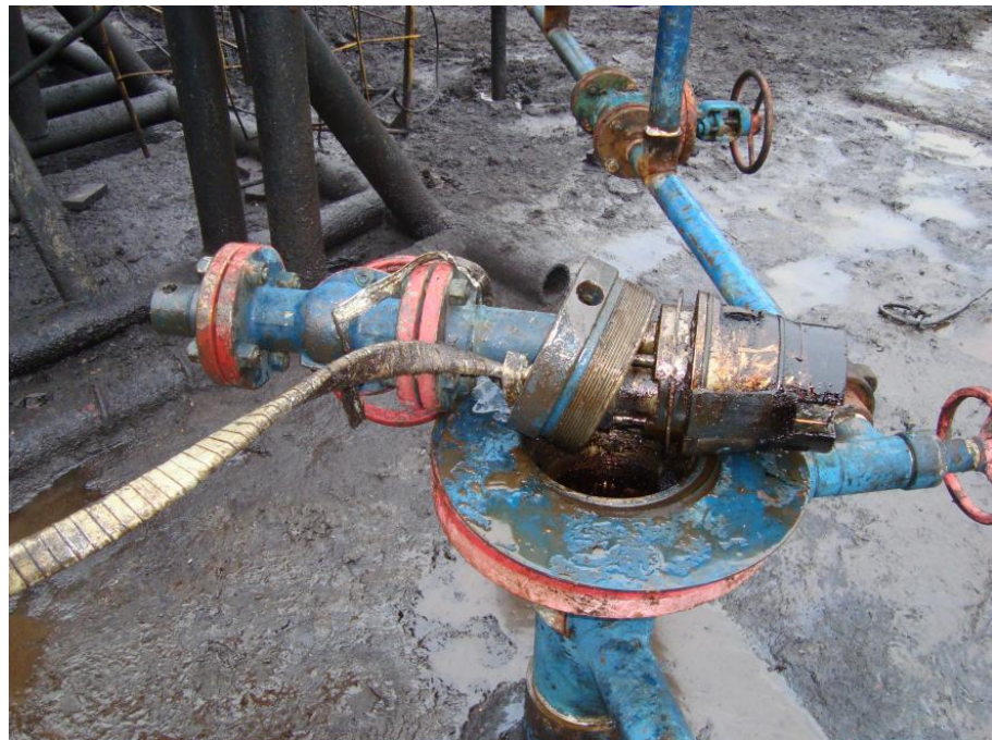
Figure 4. The fall downhole of the ESP due to the breakage of the suspension branch pipe over the body
