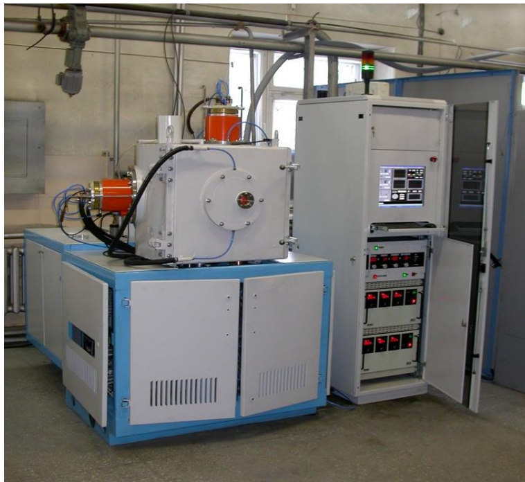
Fig.2.6 External view of the installation VNN-6
