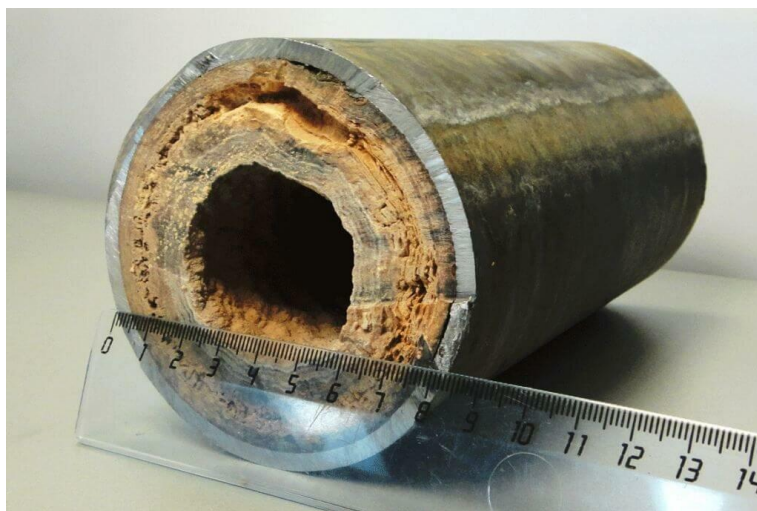
Figure 1 – Salt deposition of calcium carbonate in the pipeline
