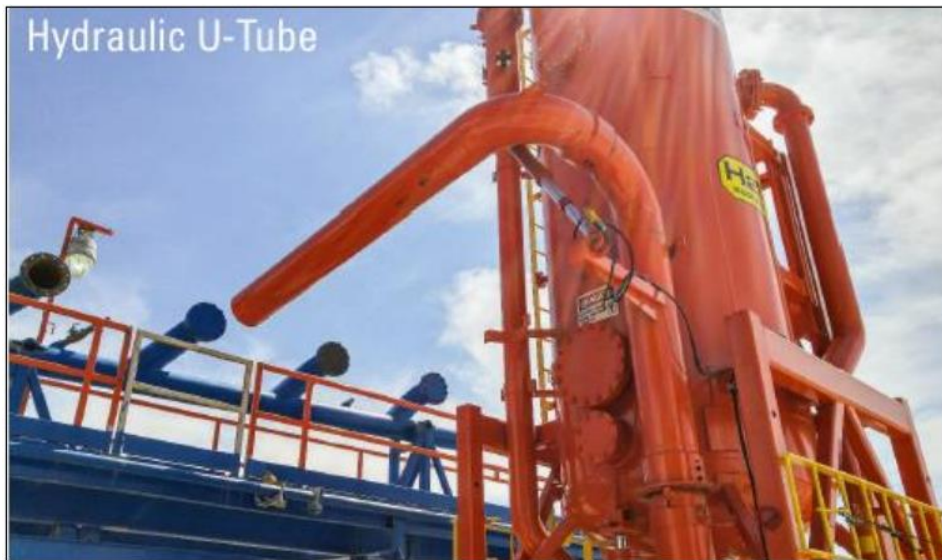
Figure 11 - MGS-Mud Gas Separator
