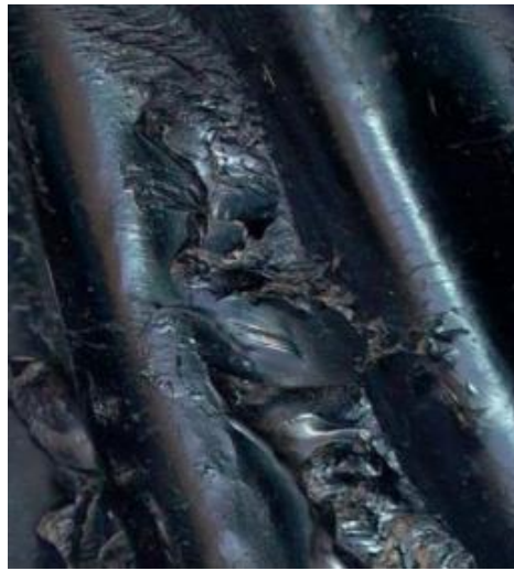
Figure 5 – destruction of the elastomer by high pressures and temperatures
