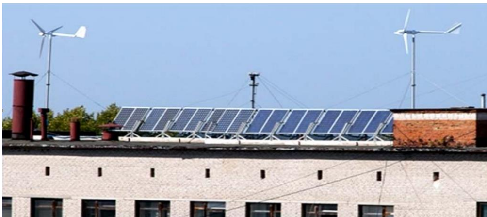
Figure 2. A view of the PV system.
