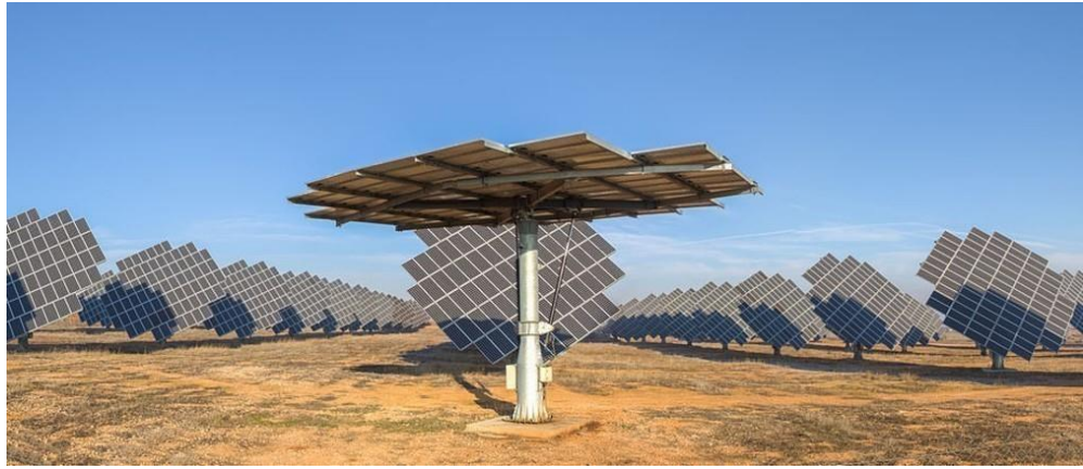
Fig. 3 A solar power plant that can track the sun
