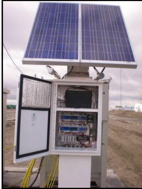
Figure 5 – Surface control unit
