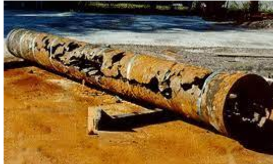
Picture 4 - example of underground corrosion
