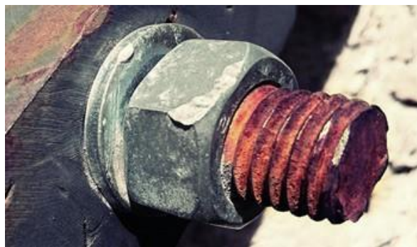
Picture 5 - contact corrosion
