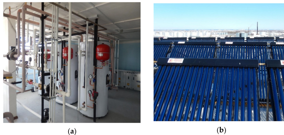
Figure 2. Engineering equipment for heat supply of apartment buildings: (a) hot water supply with one gas-fired boiler and three storage tanks; (b) arrangement of solar collectors, each consisting of 20 evacuated tubes.
