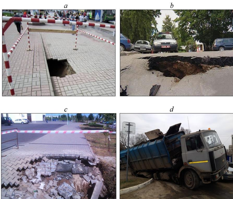
Fig. 8. Deformations of sidewalks and highways caused by suffusion: a) in Vitebsk near the Summer Amphitheater (2012); b) in Minsk along Mogilevskaya street (2014); c) in Gomel near the Ice Palace (2013); d) in Zhlobin near gymnasium no. 1 (2014) [10]
