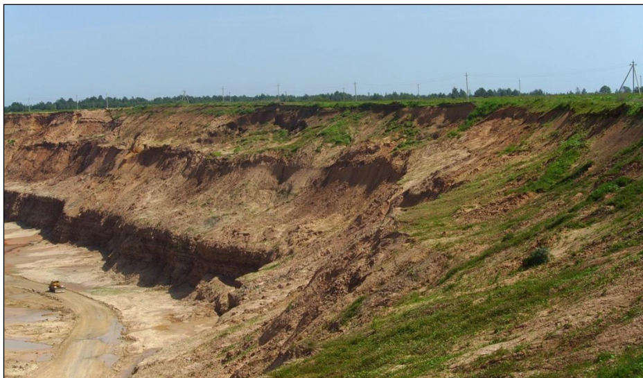
Fig. 3. Southern wall of the Galevo open pit for dolomite mining with numerous rockfall-landslide areas (May 2010). Photo by A.N. Galkin
