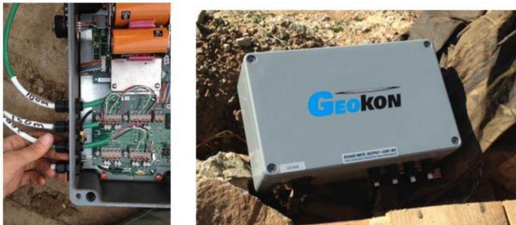
Figure 3-17: Logger for logging the data from sensors
