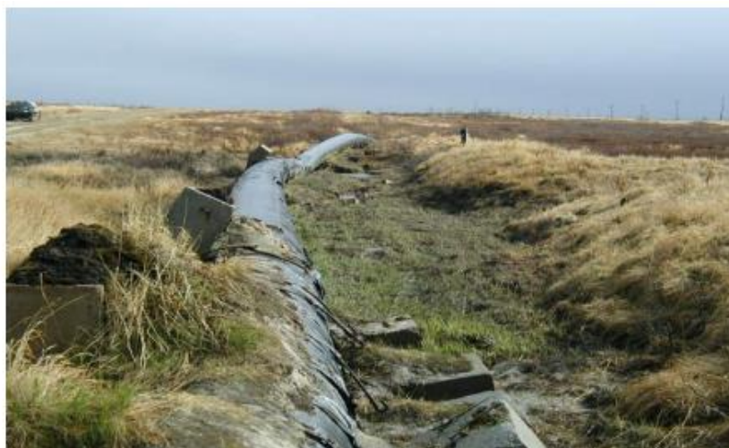
Figure 11. Surfacing of underground pipeline due to melting of permafrost soil
