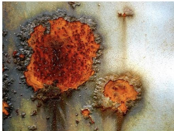
Figure 3 – Corrosion on steel surface
