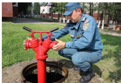
Figure 5 – External fire water supply
