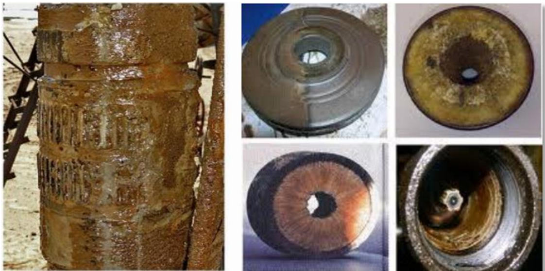
Fig. 1 Salt treatment of deep pumping equipment
