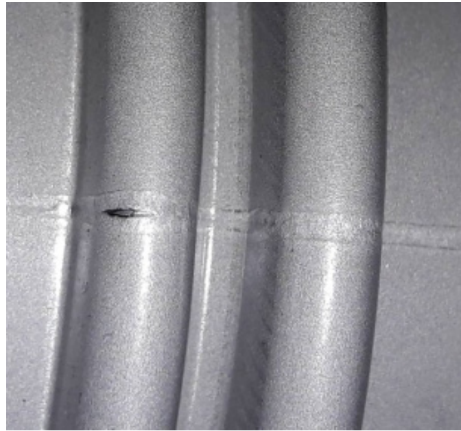
Figure 1. Destruction of the bellows expansion joint along the axis of the weld.
