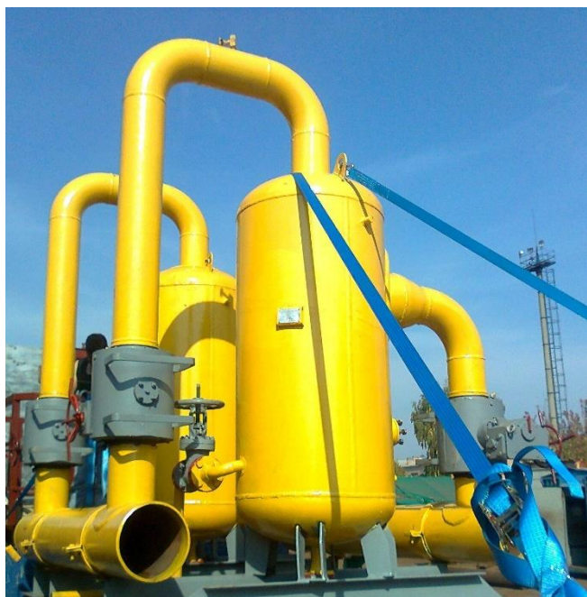
Picture 3 – Gas filter
