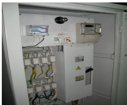
Figure 3.1.4–Mounted appliance AMR accounting system
