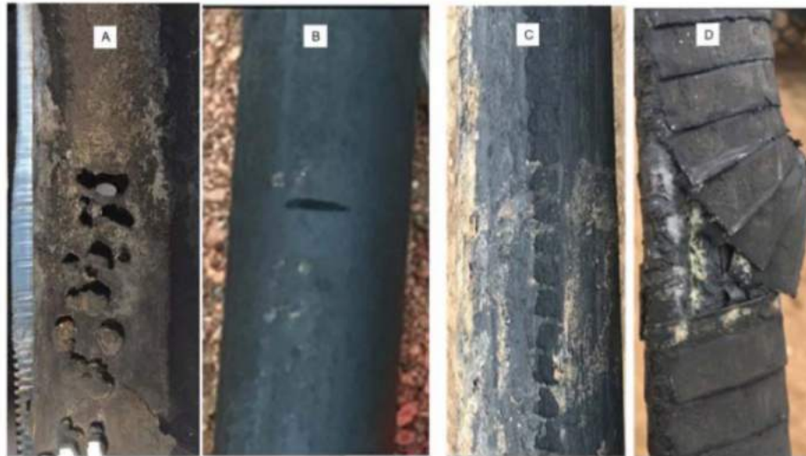
Figure 2—Examples of corrosion challenges to ESP well: A) internal tubing corrosion, B) external tubing corrosion, C) tubing scale and cable armor corrosion, D cable armor corrosion
