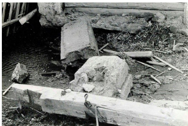
Photo 1. The left concrete column is broken in half and thrown to the left. On the right, its lower part is visible (Photo by Fefelov V. N.)
